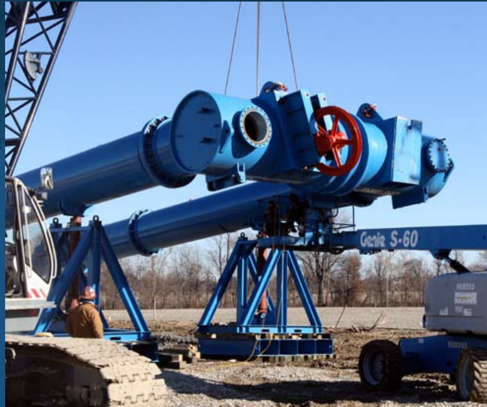
FKCI's Blind Drilling crew works on preparations for raising the DHI 240's mast at the Oaktown Shafts Project (FKCI Job No. 08.17) in late December.
